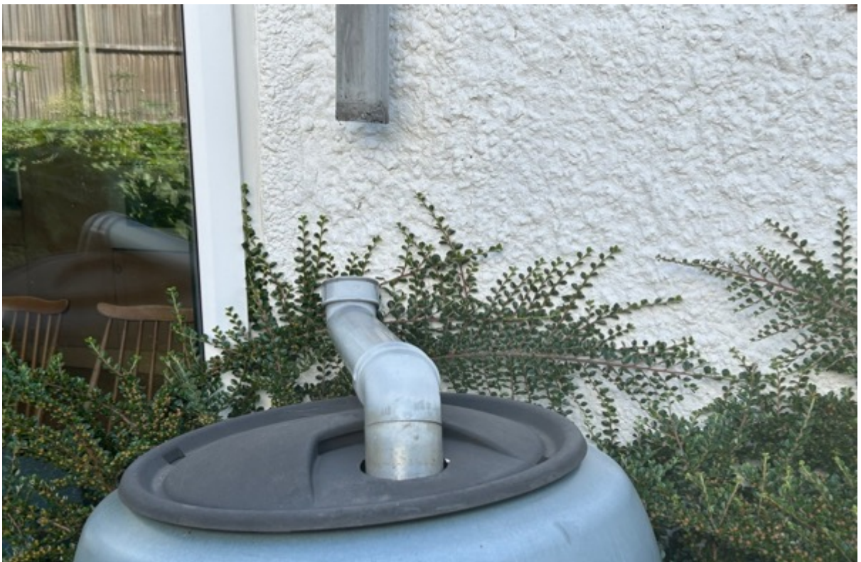
Separated downpipe to the left side of the property.
