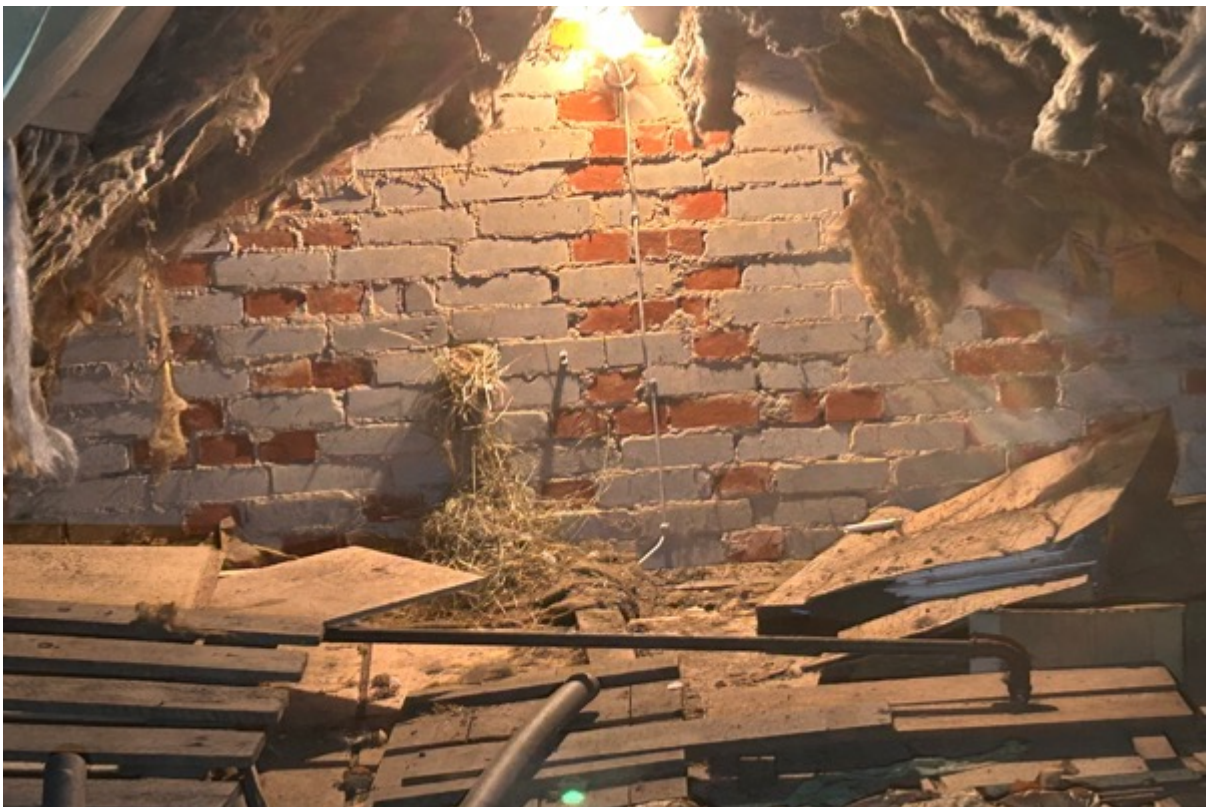
Rear of the main roof an utter mess (2).
