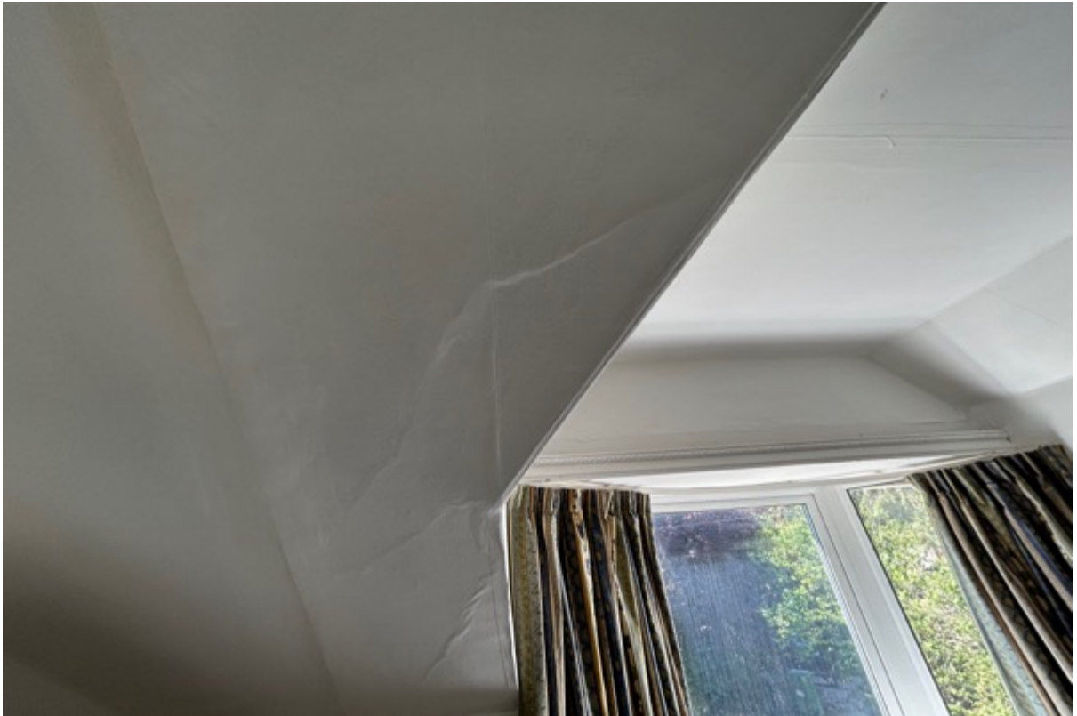
Example of cracking to the lath and plaster ceiling to the front right bedroom.
