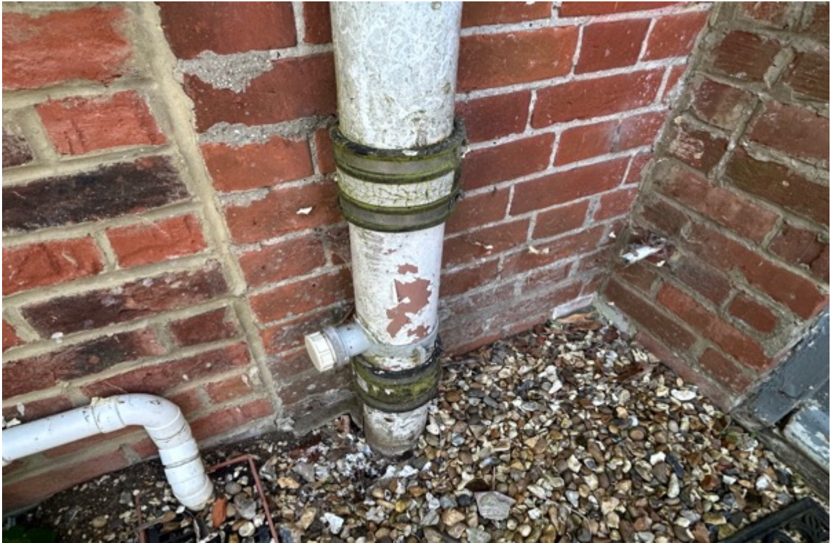
Perishing jubilee clips to the rear soil stack.
