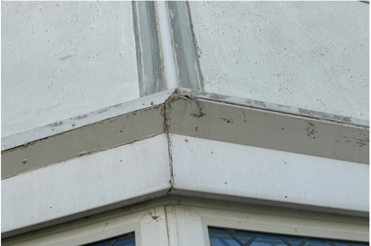
Poorly jointed PVC trim to the bay to the left side of the property.
