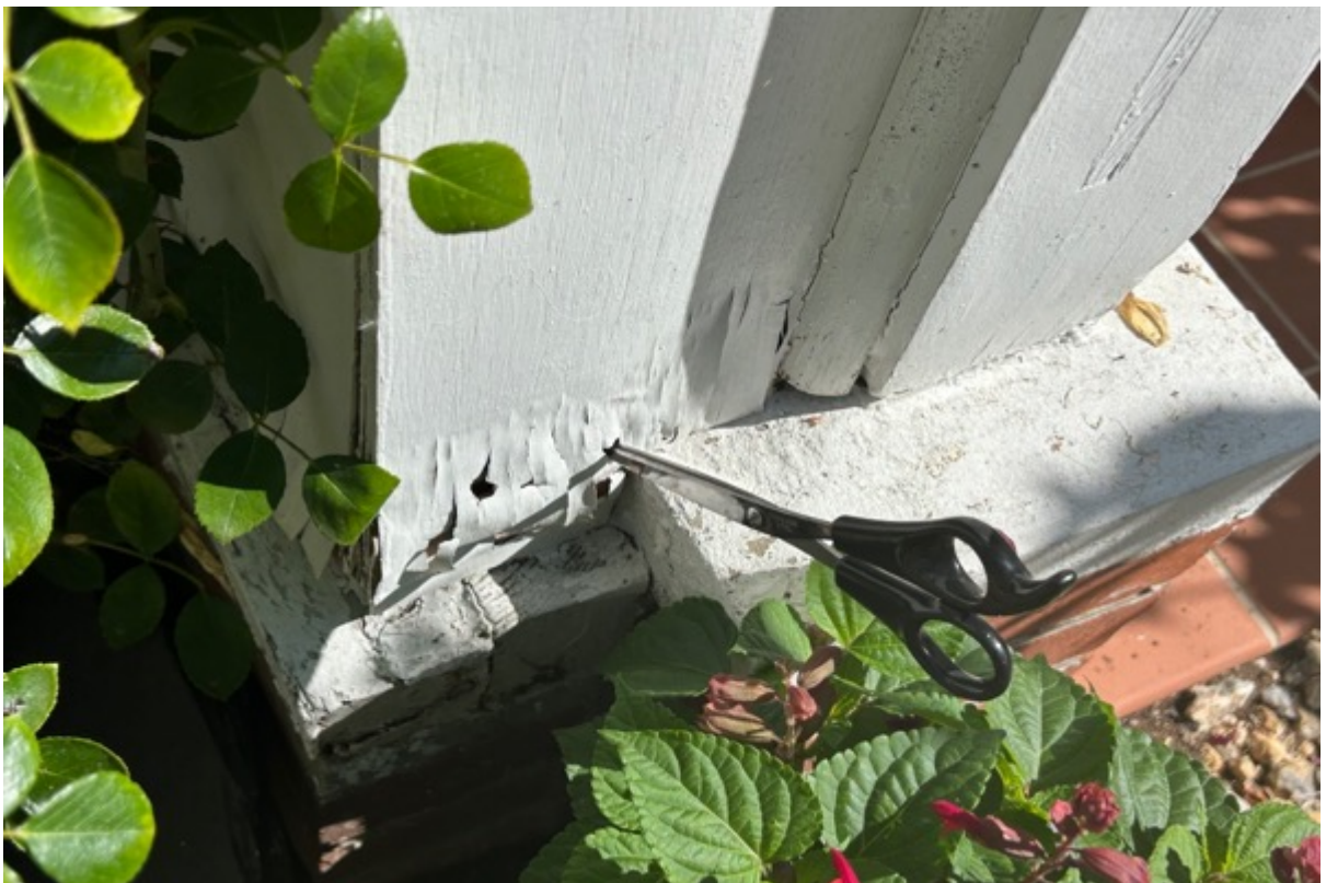
Timber decay to the front porch joinery (2).
