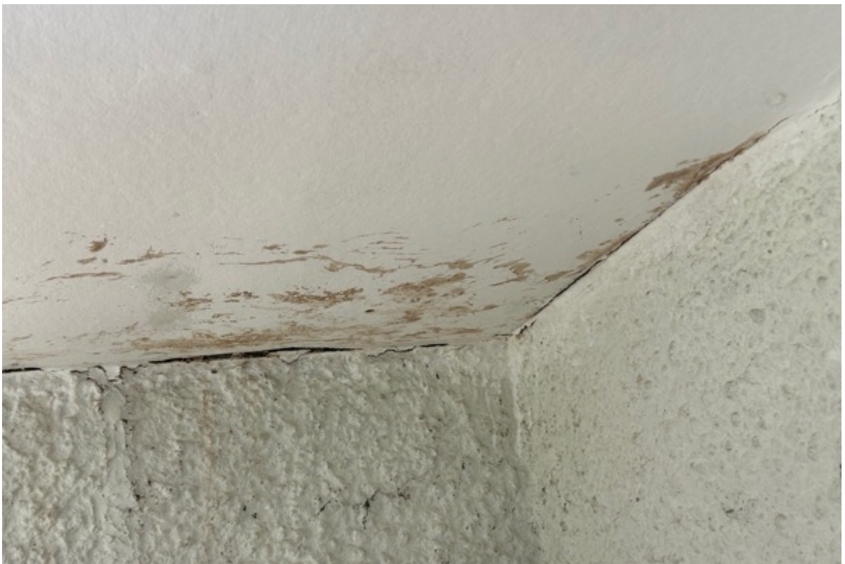
Severe damp staining to the ceiling to the garden room (1).
