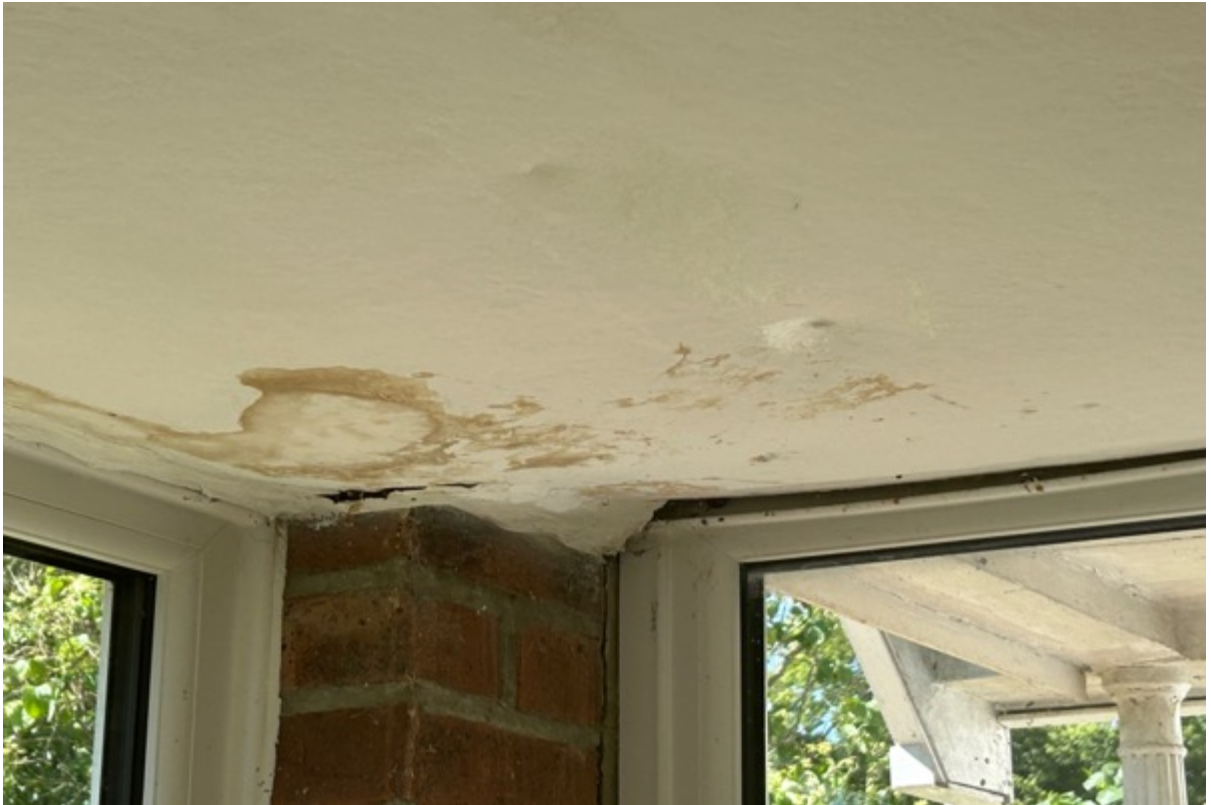
Severe damp staining to the ceiling to the garden room (2).
