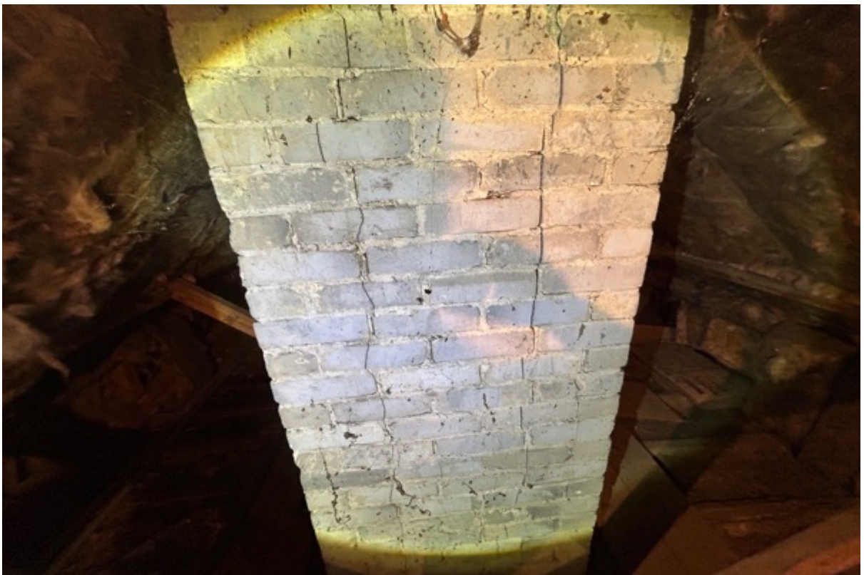
Hairline cracks to the roof space chimney breast.
