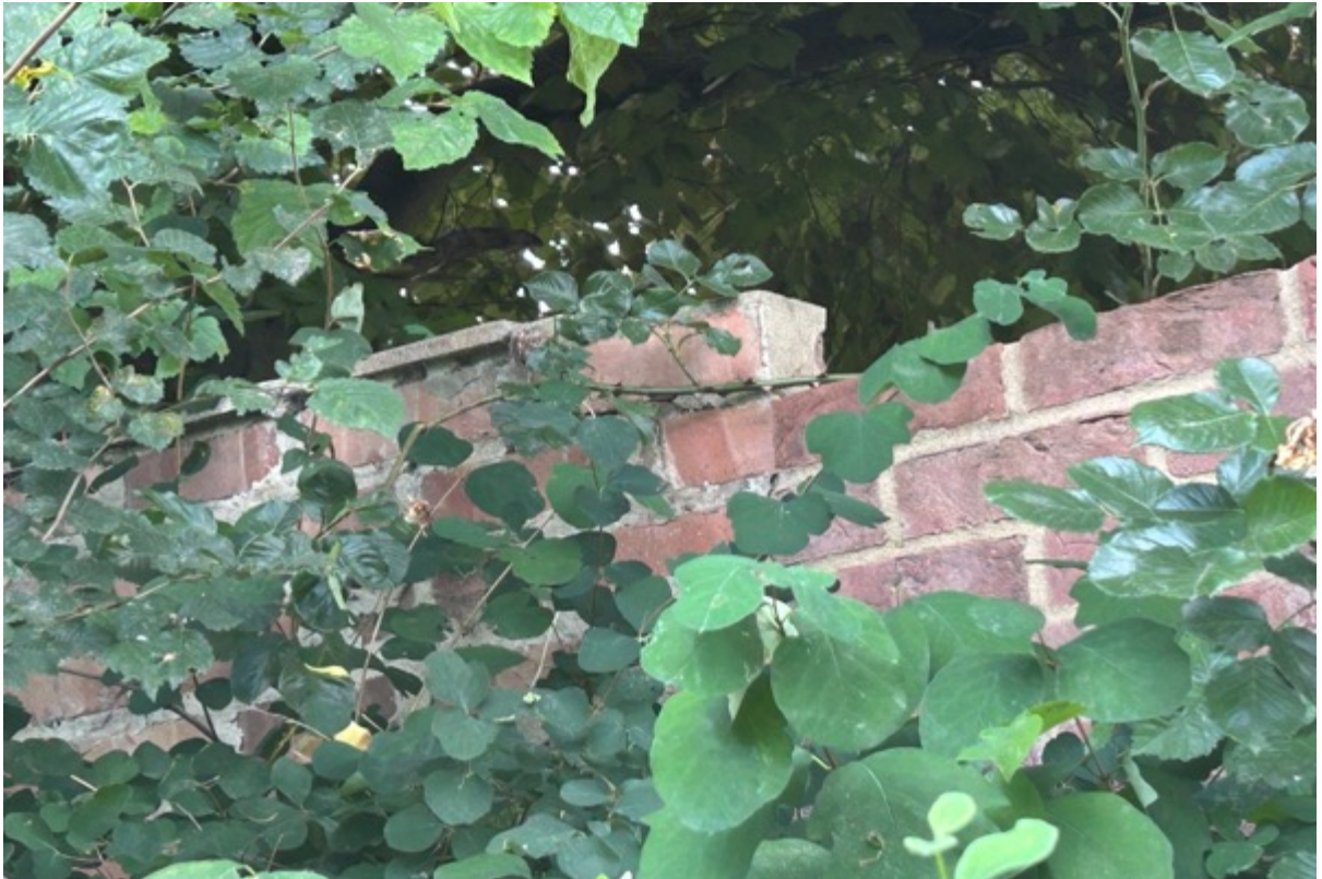
Damage to the boundary wall to the right side of the garden (1).
