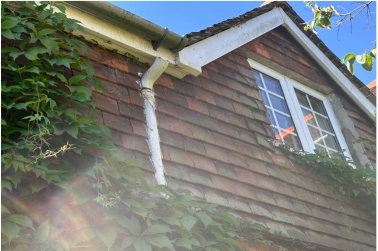
What appears to be an old, redundant pipe embedded in the tile hanging to the rear of the property.
