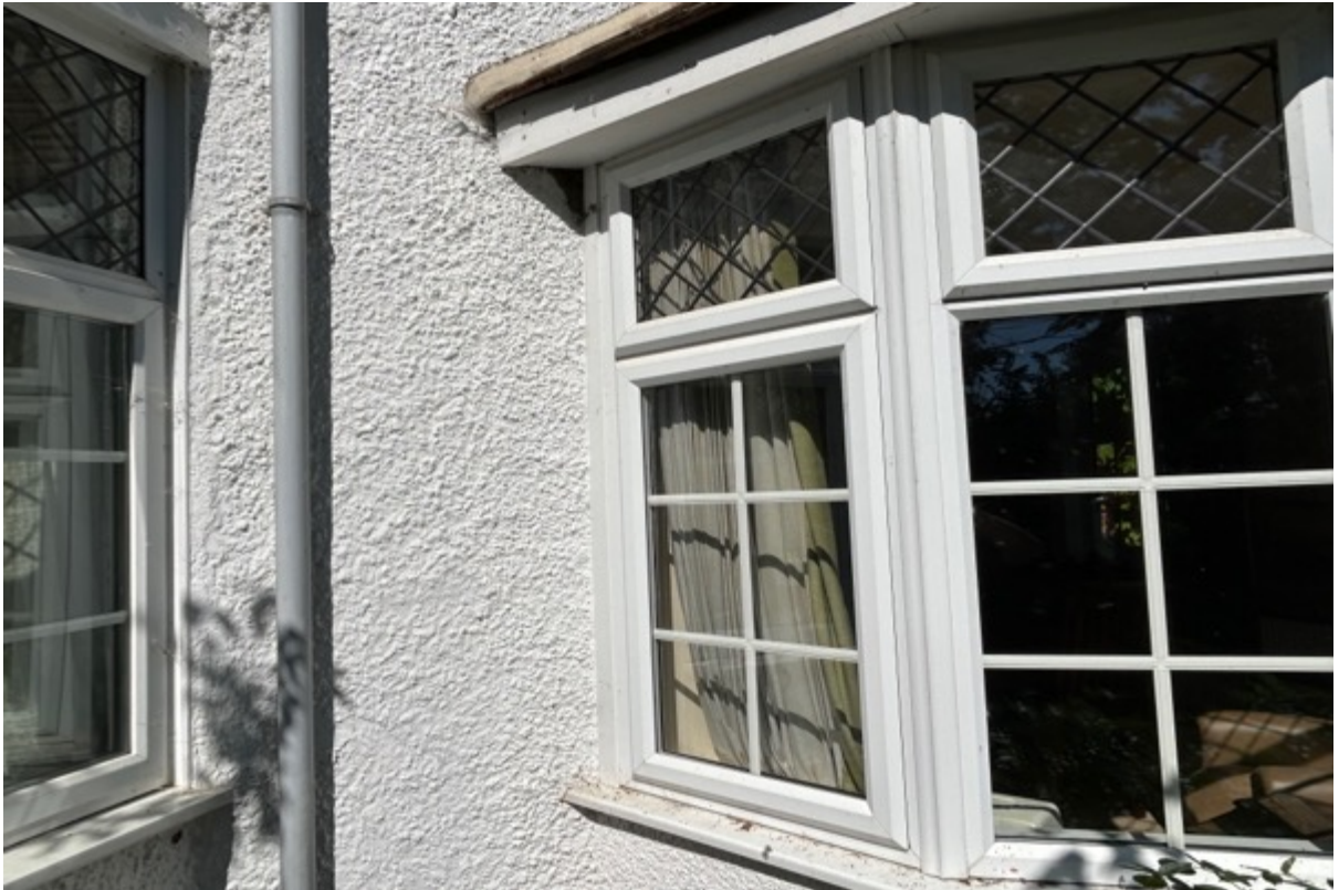
No separation between the left side of the adjacent, smaller bay and the right flank elevation.
