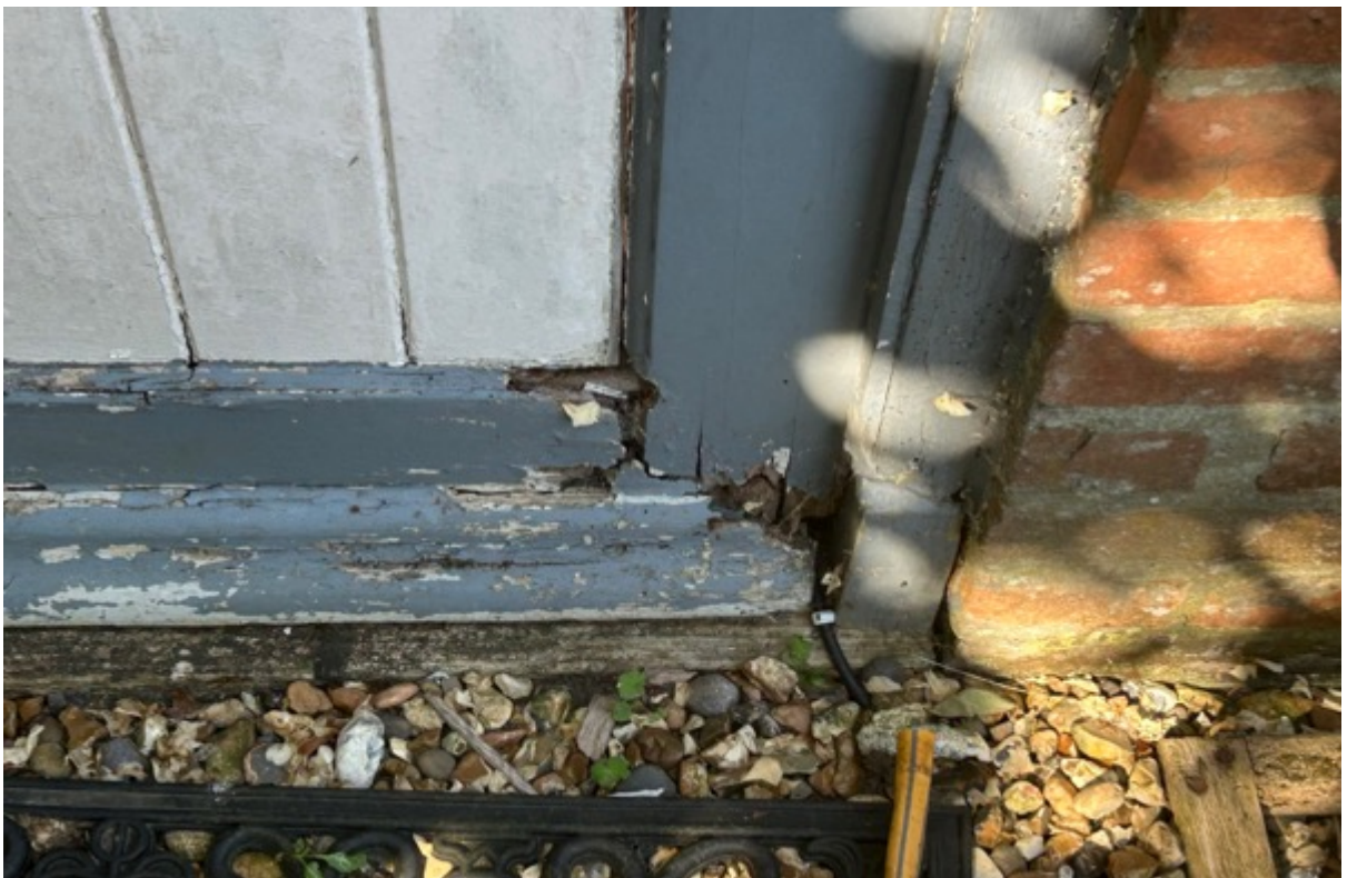
Severe timber decay to the right side door to the Perspex sheeted enclosed area to the rear of the property.
