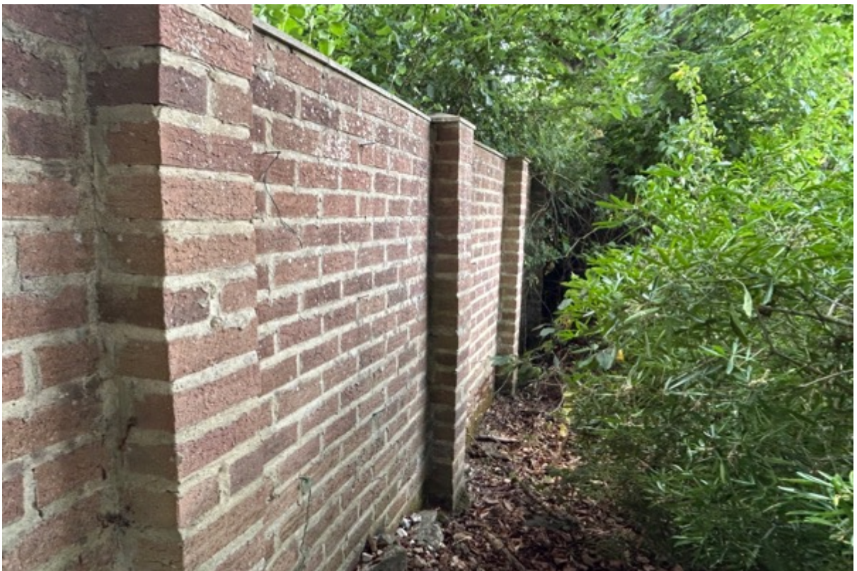
Right side boundary wall showing the first signs of leaning.
