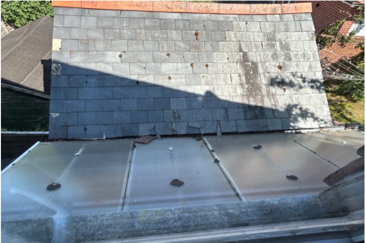
Front slated slope to the same outbuilding, with a number of the slates damaged.
