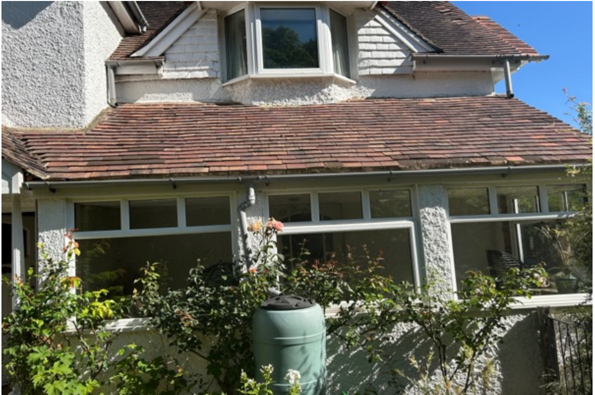
General view of the garden room roof, with significant unevenness to the roof profile.
