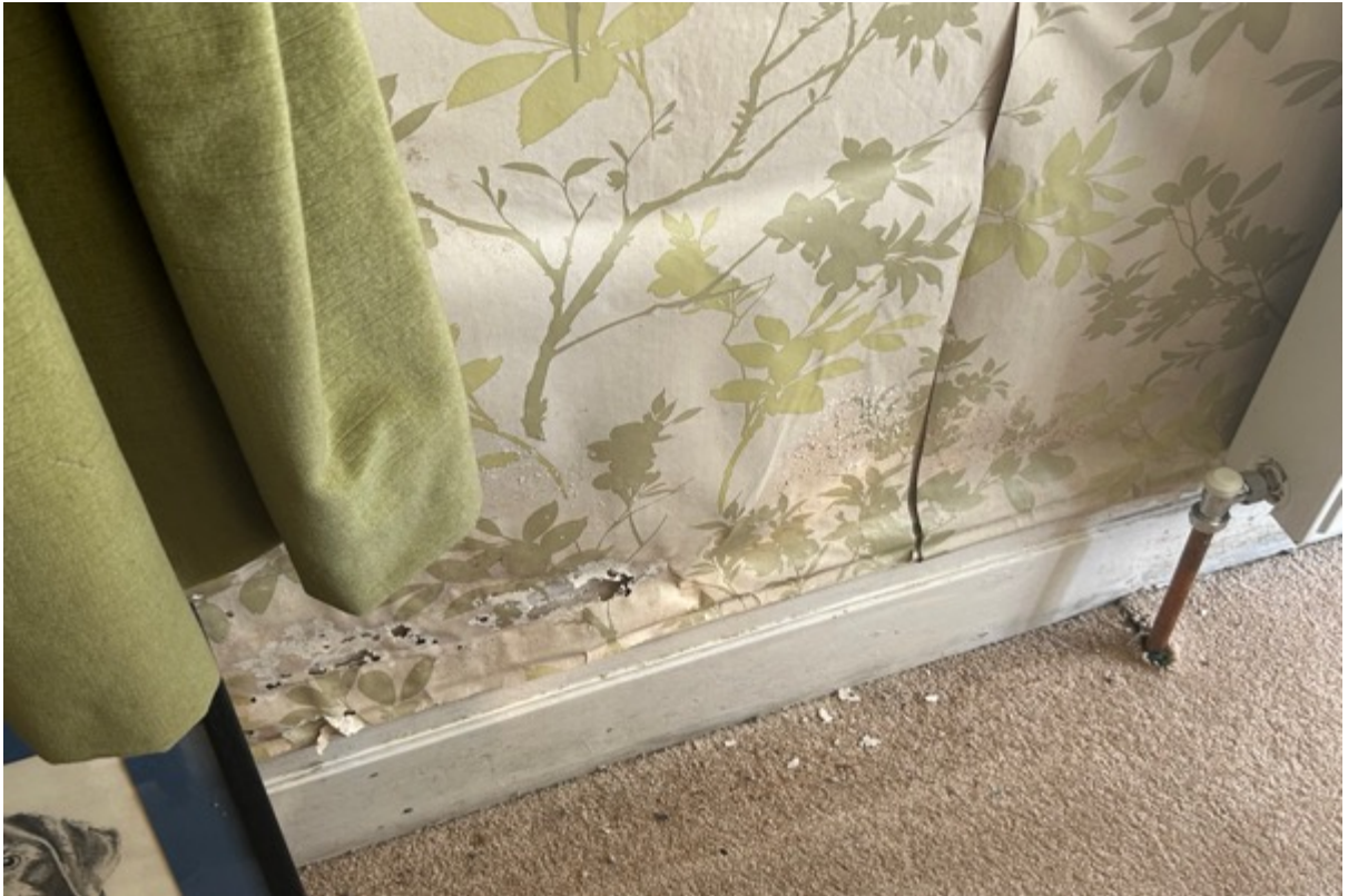
Severe rising damp to the rear wall of the main right side reception room (2).
