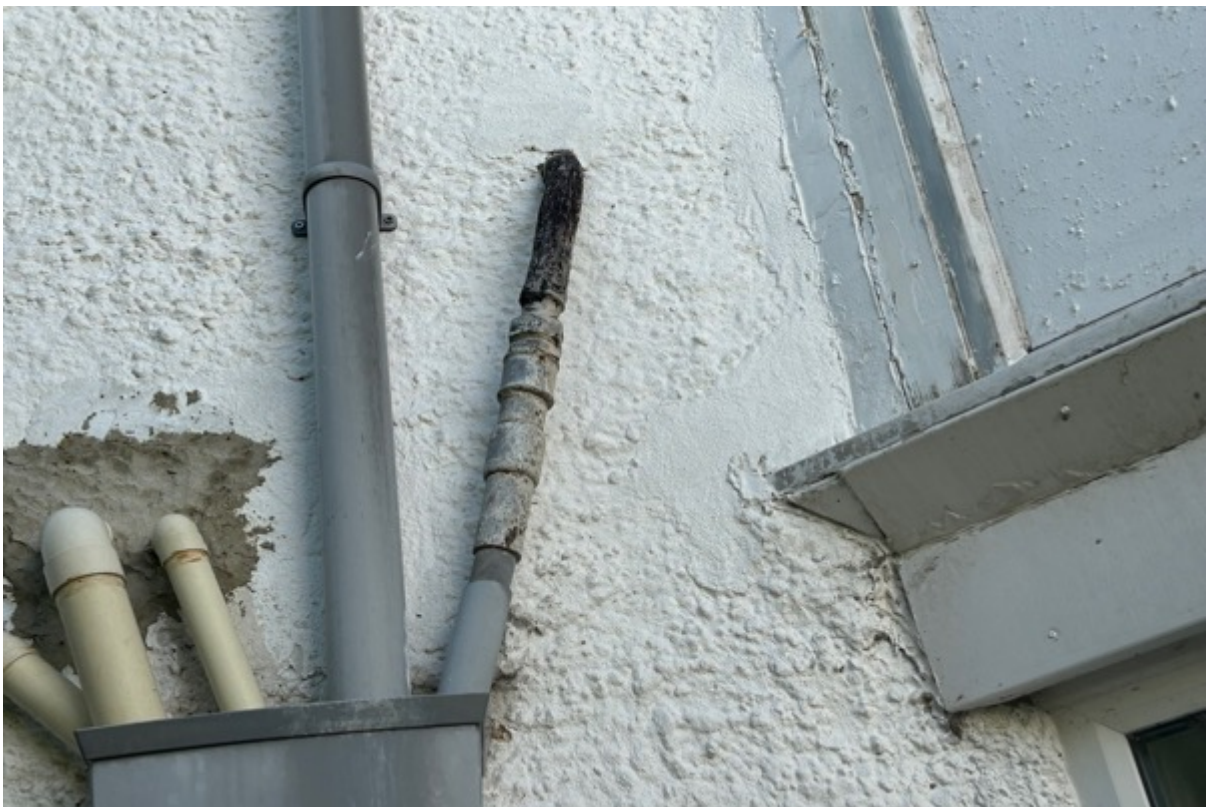
Example of an old, corroding waste pipe coming out through the render to the left flank elevation.
