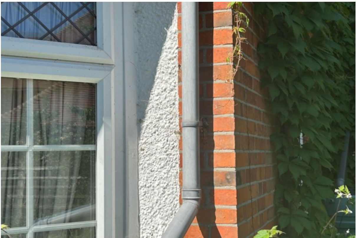
No separation between the right side of the adjacent, smaller bay and the right flank elevation.
