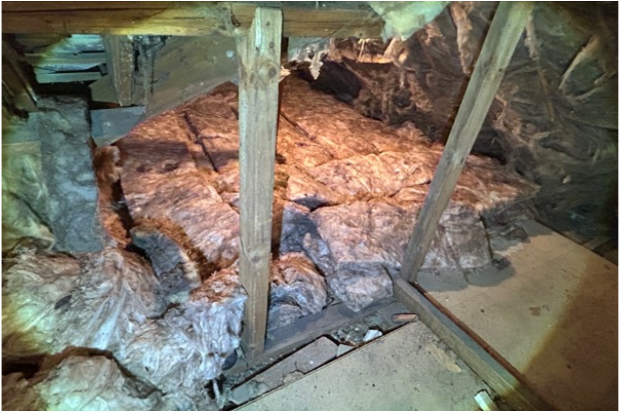
Fibre insulation quilt haphazardly piled across the ceiling joists in one area.
