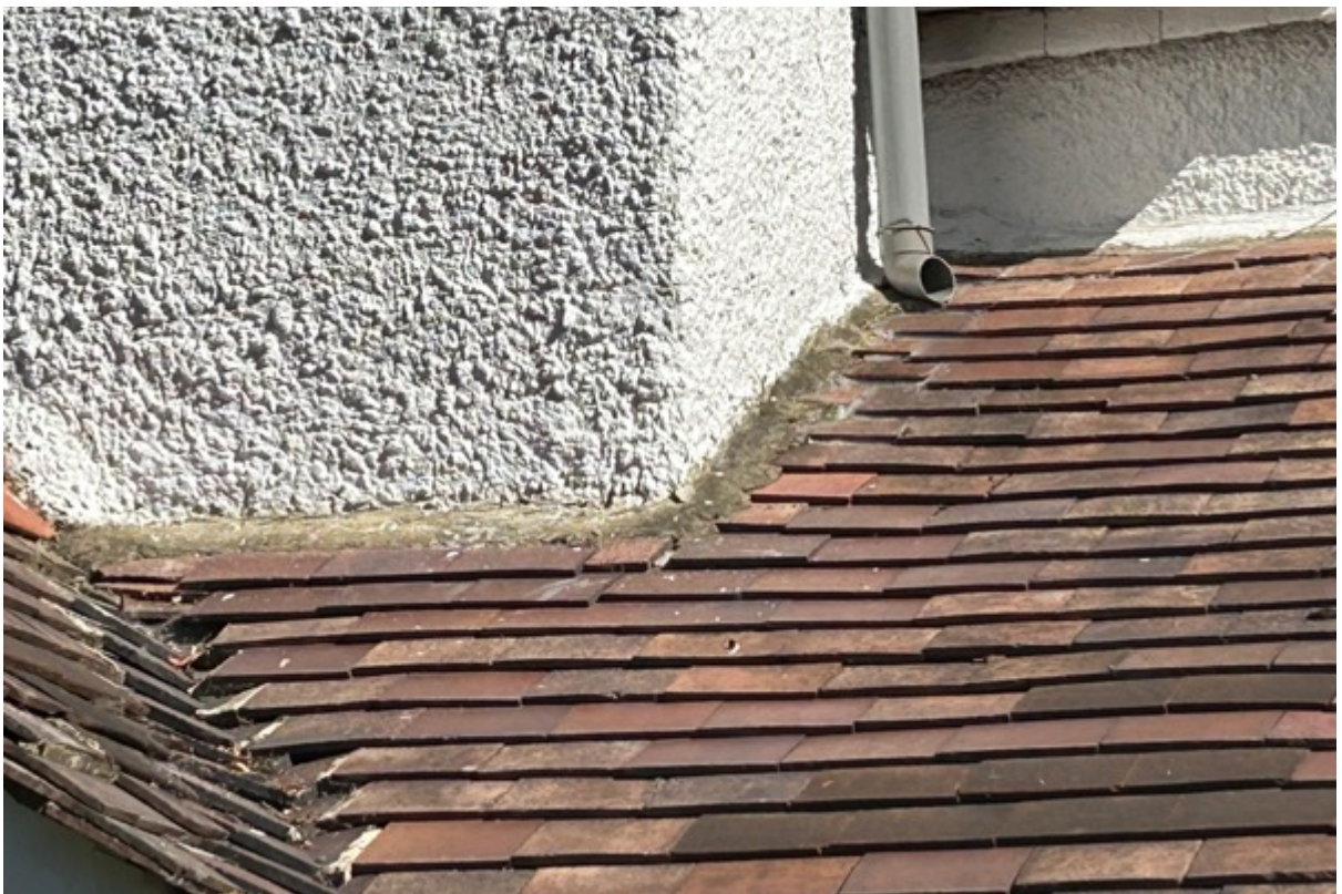
Inadequate cement fillet waterproofing the perimeter of the same roof (1).
