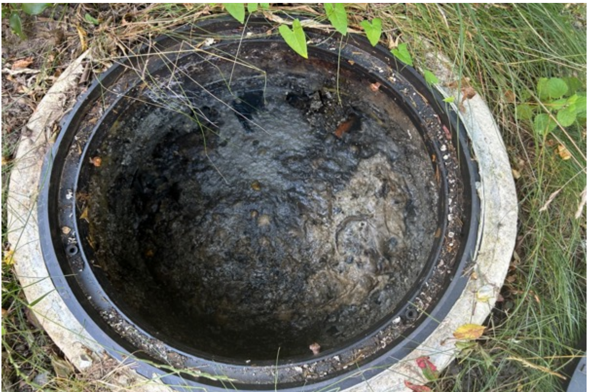
Inspection chamber full to the top with effluent.
