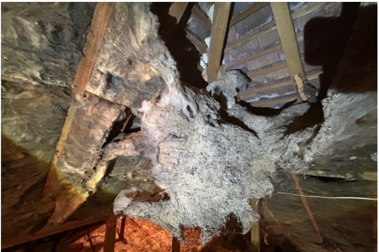
Fibre insulation quilt between the rafters heavily dirt contaminated and coming out of position.
