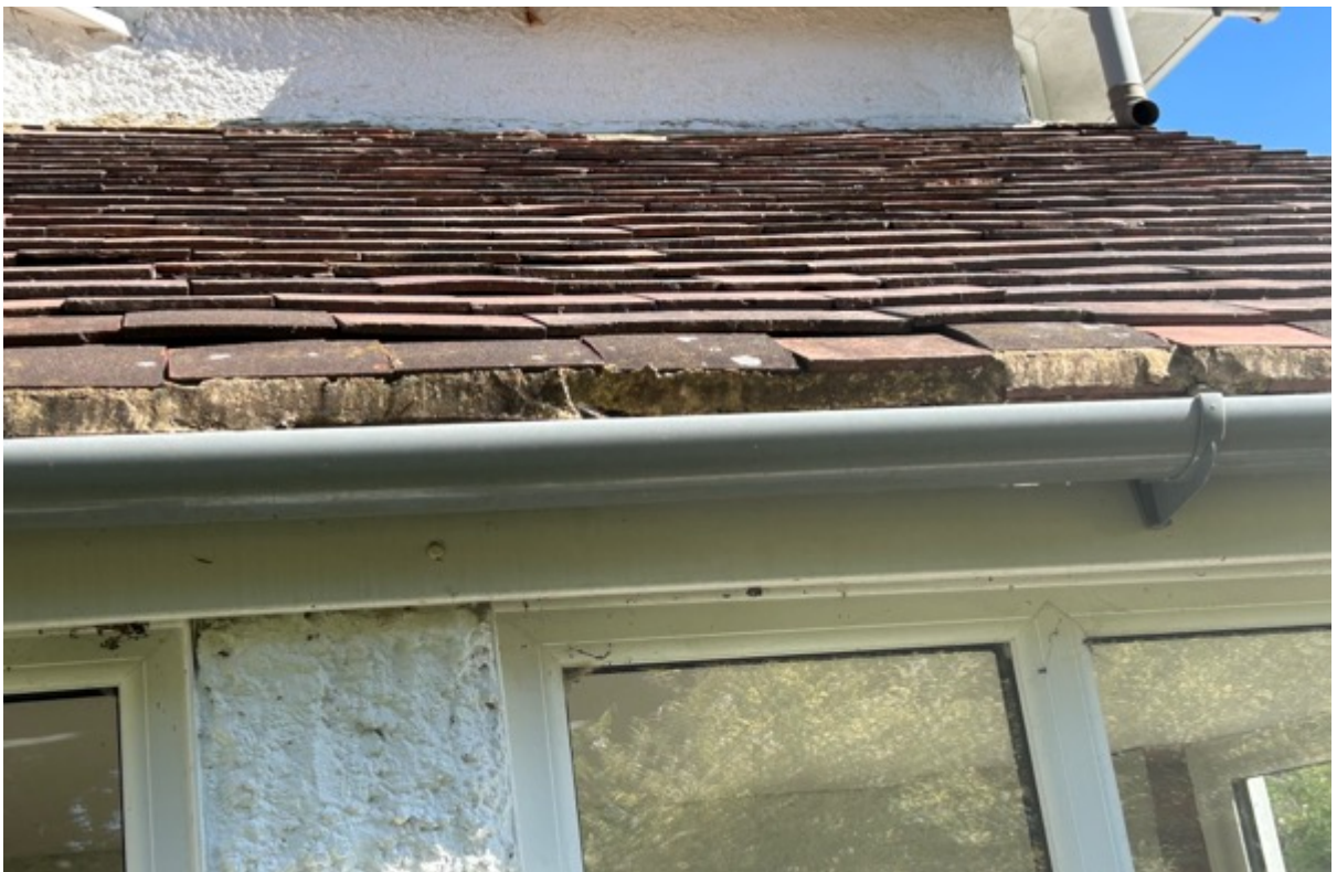
Bizarre arrangement to the bottom of the tiles, with a mortar infill rather than a projecting strip of sarking felt.
