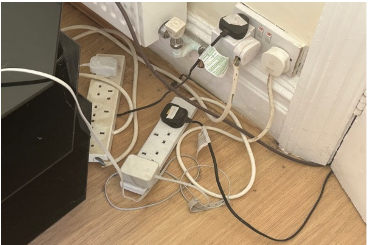
Confirmation that the property has an inadequate number of socket outlets.
