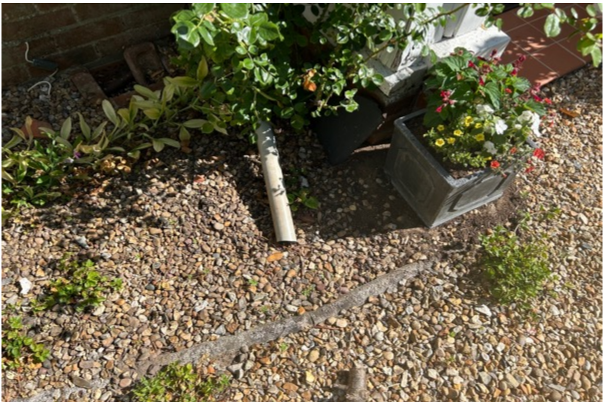
Front rainwater downpipe simply discharging onto the shingle.
