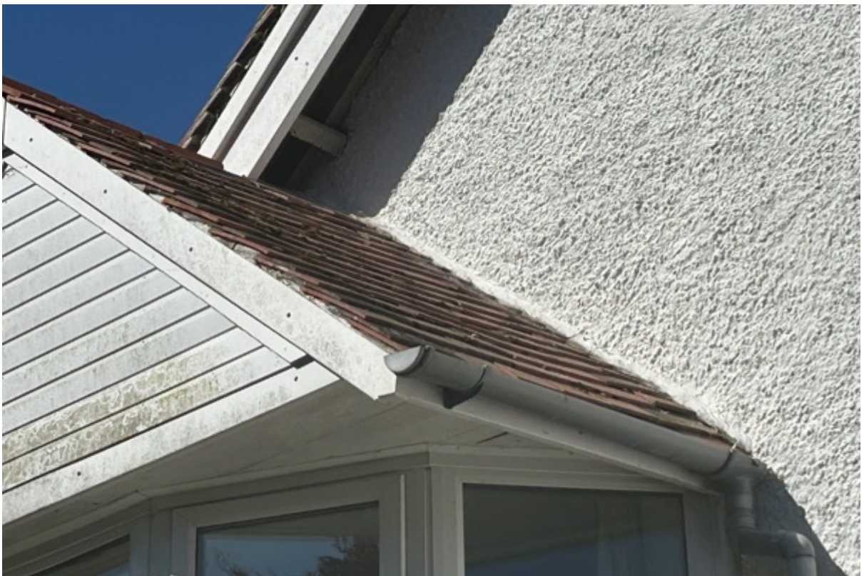
Poor quality waterproofing arrangement to the left side of the rear slope to the same roof.
