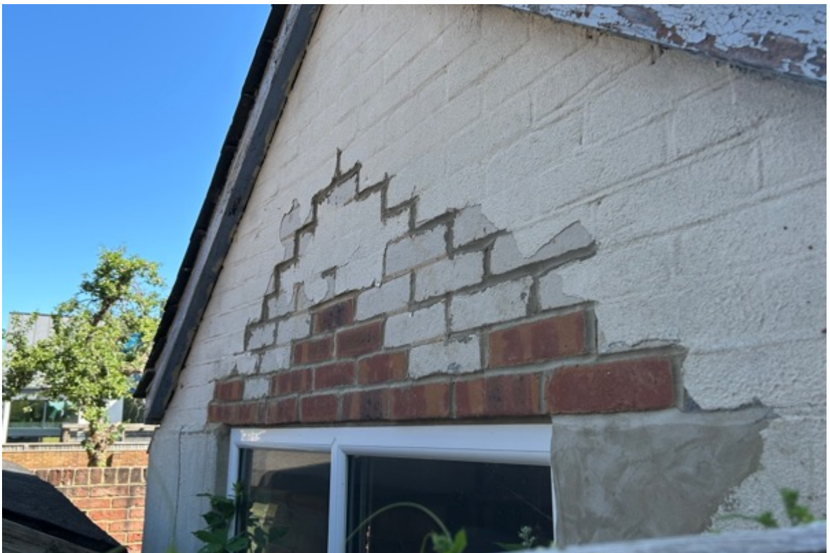
Inadequately supported brickwork above the left side window opening to the same rear shed.
