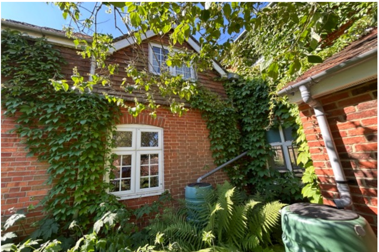
Significant creeper growth obscuring areas of the rear of the property.
