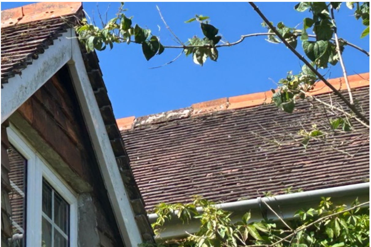
Several badly weathered, non-matching ridge tiles to the rear of the main roof.
