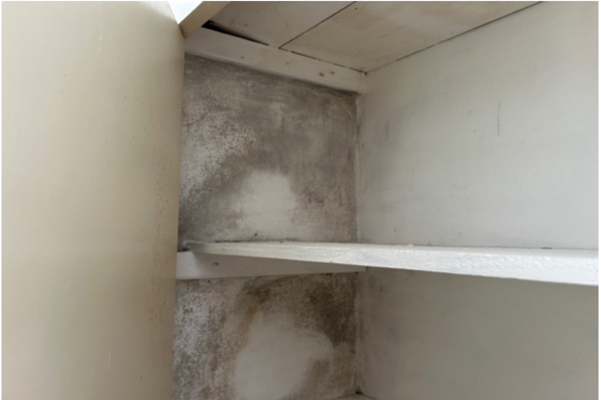
Example of mould staining to one of the built-in cupboards (2).
