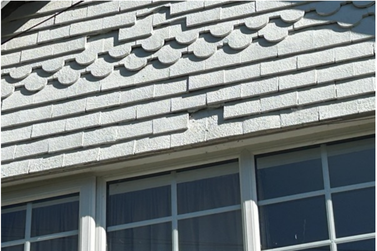
Missing tile at high level to the front gable tile hanging.
