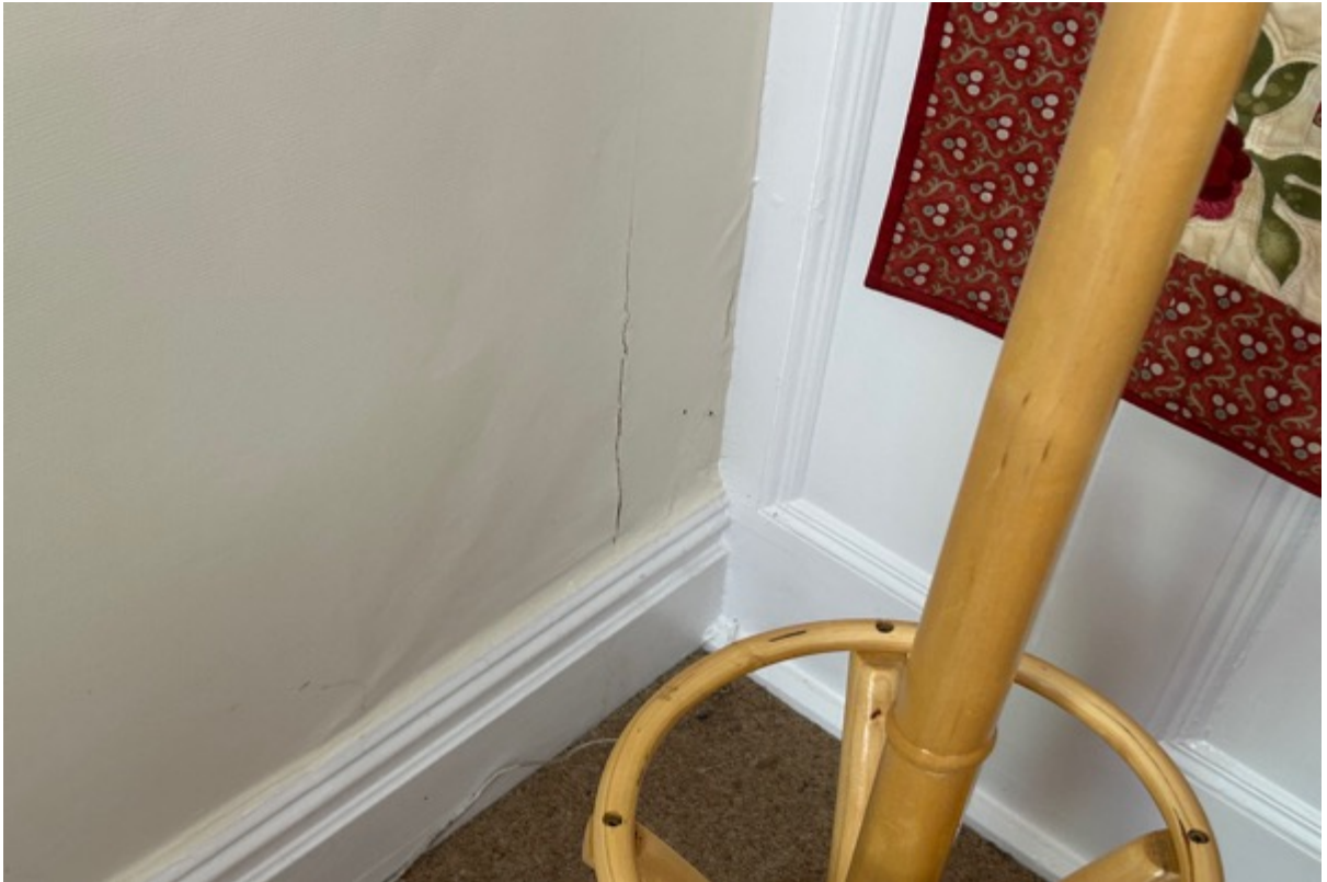
Area of rising damp to the rear left corner of the front lobby/reception room.
