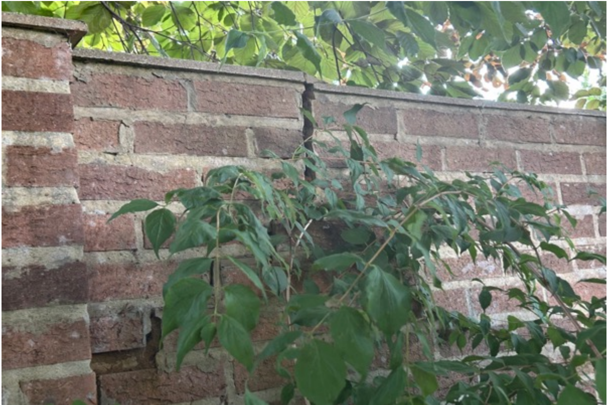
Damage to the boundary wall to the right side of the garden (3).
