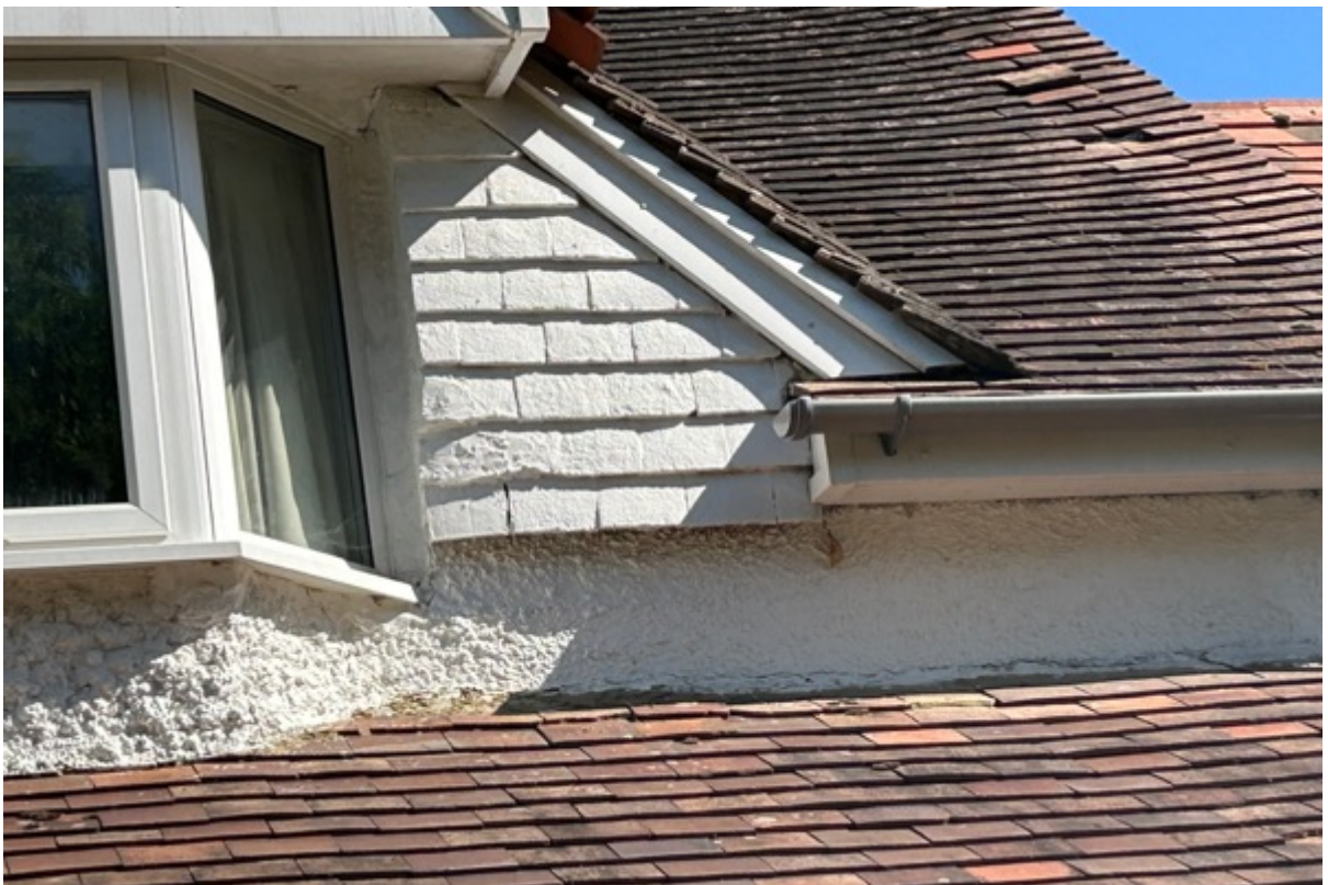
Several tiles to the area of painted file hanging badly profiled and needing replacement.
