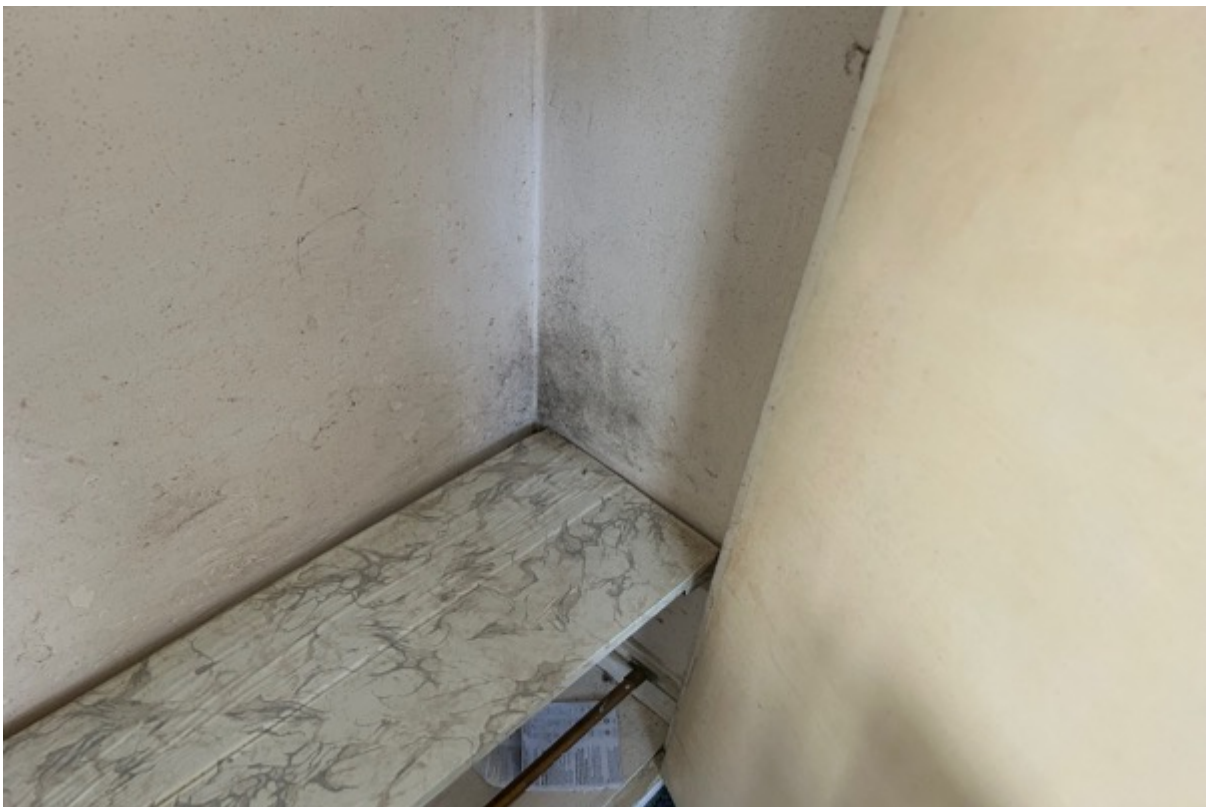
Example of mould staining to one of the built-in cupboards (1).
