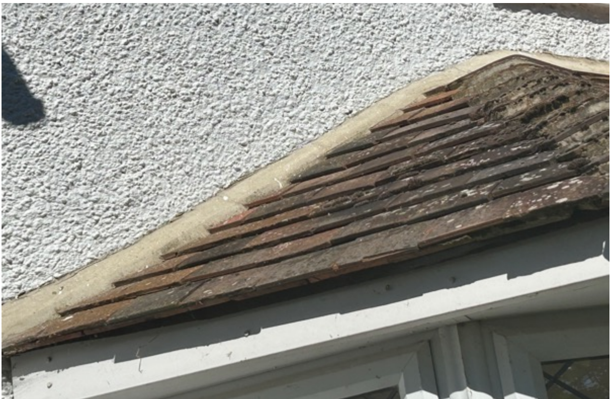
Poor quality cement fillet waterproofing the joint between the same roof and the right side elevation roughcast render.
