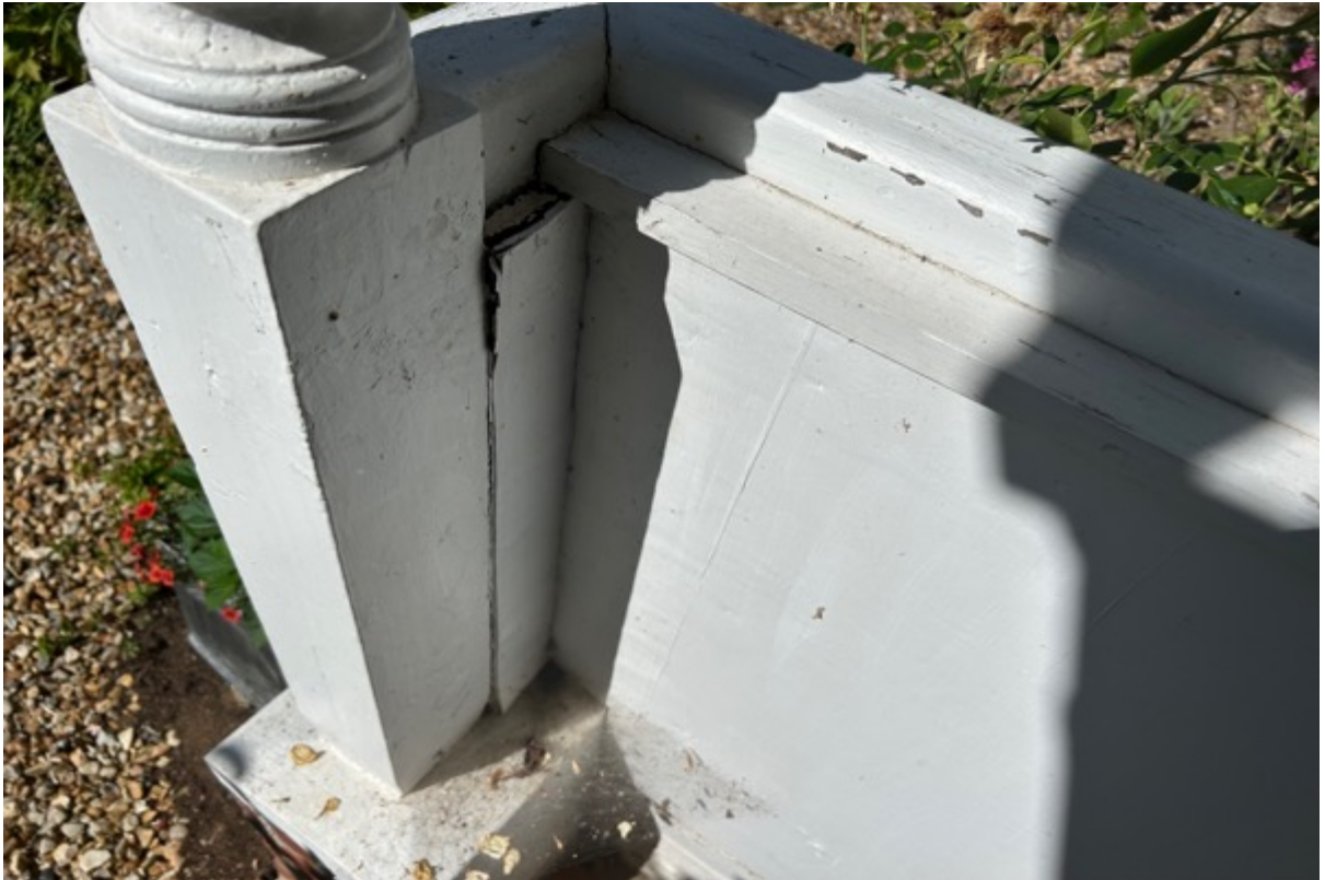
Timber decay to the front porch joinery (1).
