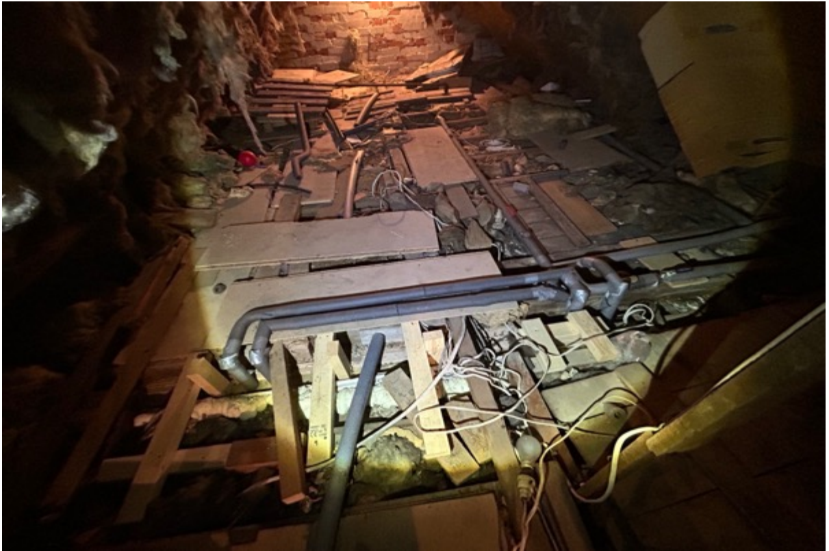
Rear of the main roof an utter mess (1).
