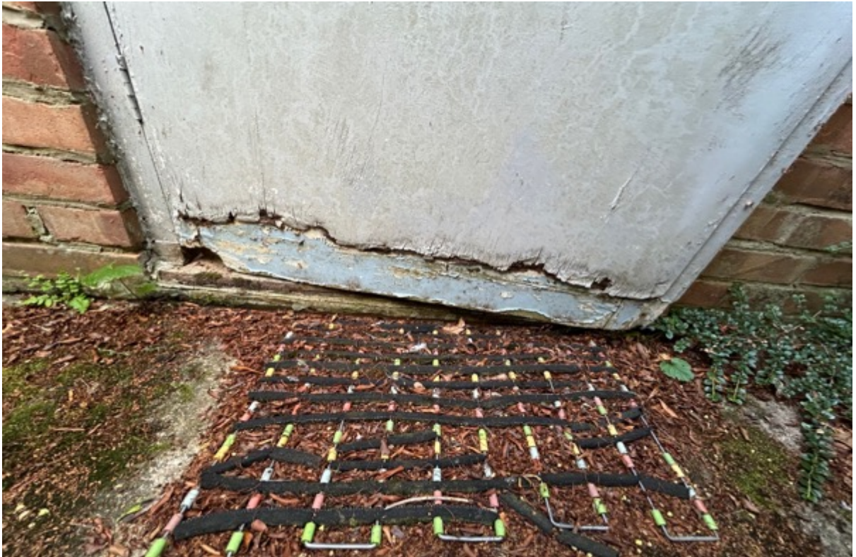
Severe timber decay to the second door to the Perspex sheeted enclosed area to the rear of the property.
