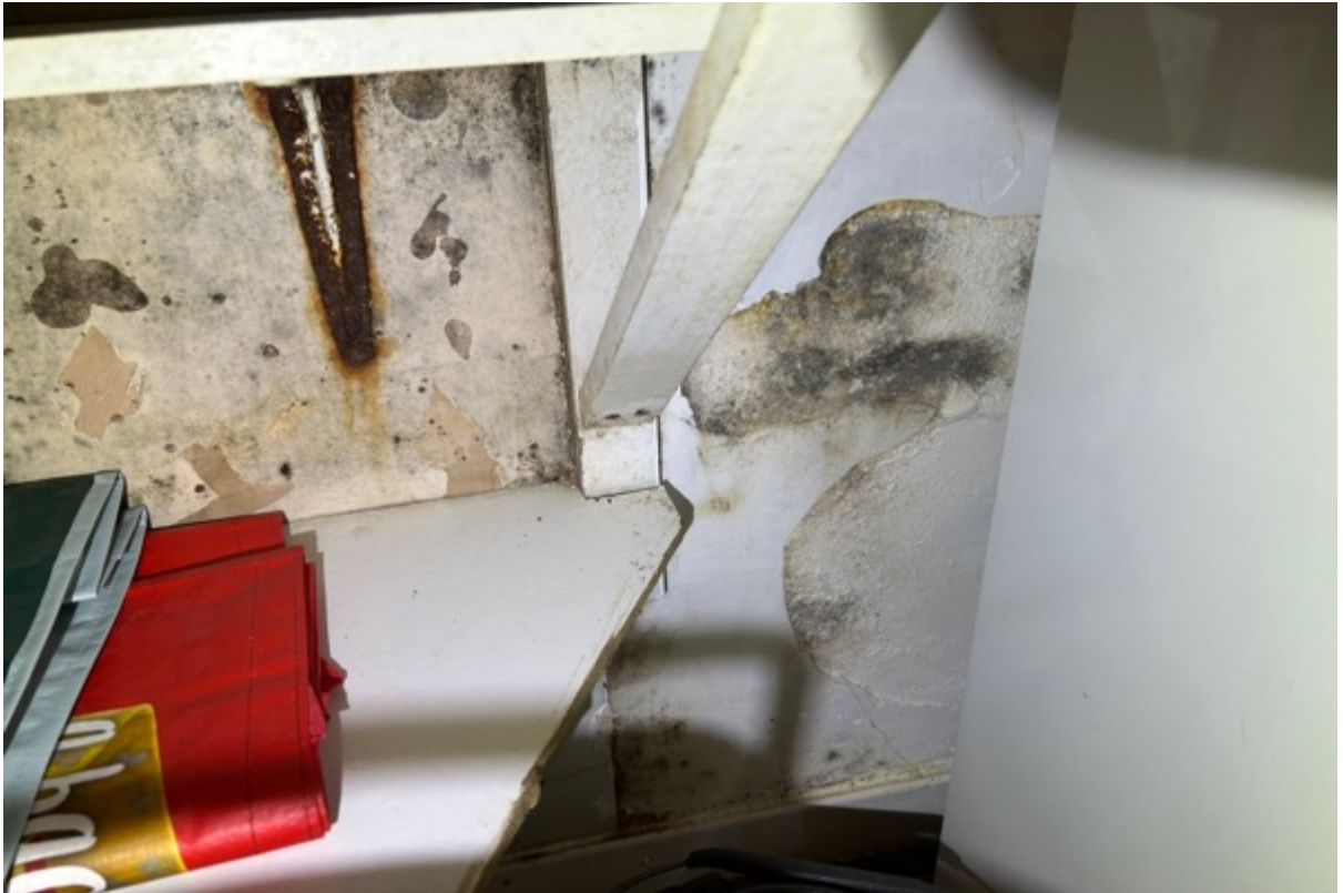
Rising damp to the left side wall to the utility room.
