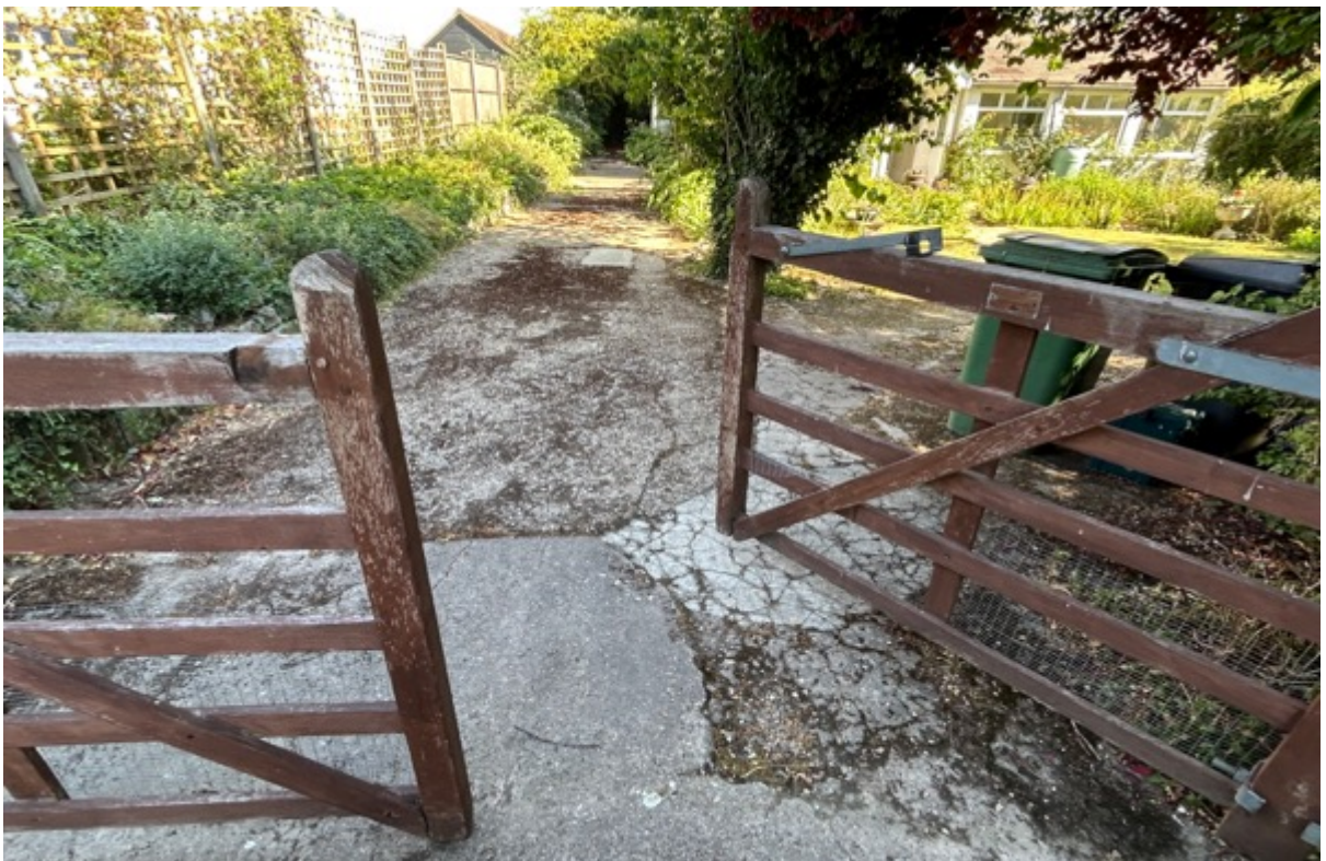
Front gates badly weathered and no longer meeting properly, with the concrete to the driveway beyond in poor condition.
