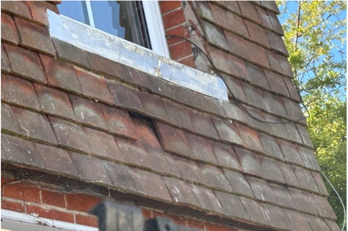
Missing tile to the vertical tile hanging to the rear of the property.
