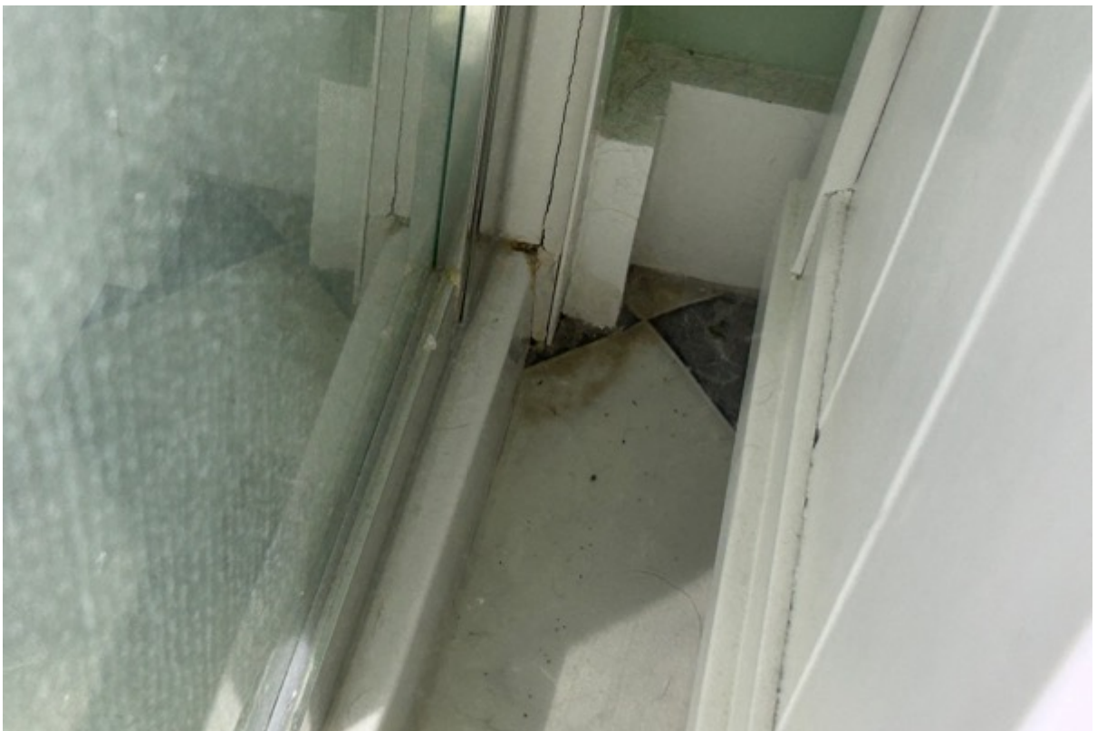
Clear leakage to the first floor bathroom shower enclosure.
