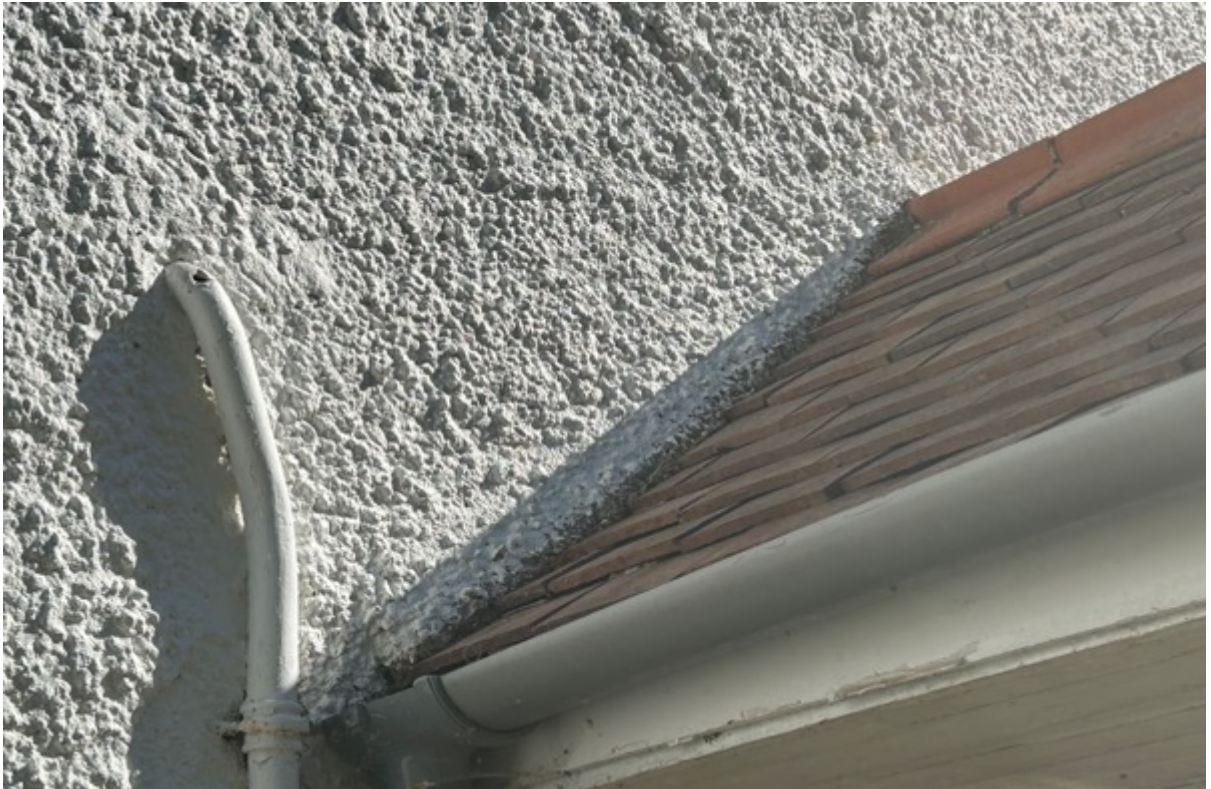
Inadequate cement fillet waterproofing the perimeter of the same roof (2).
