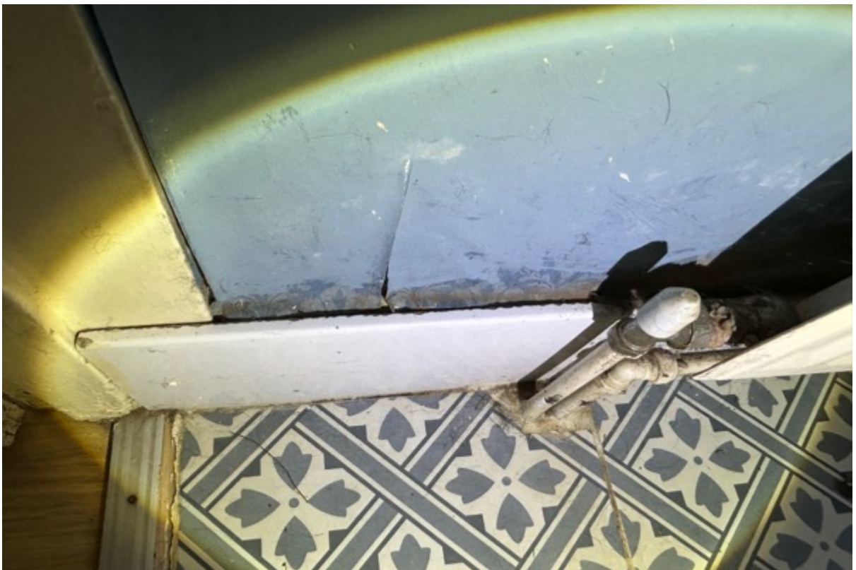
Rising damp to the left side wall to the rear lobby.
