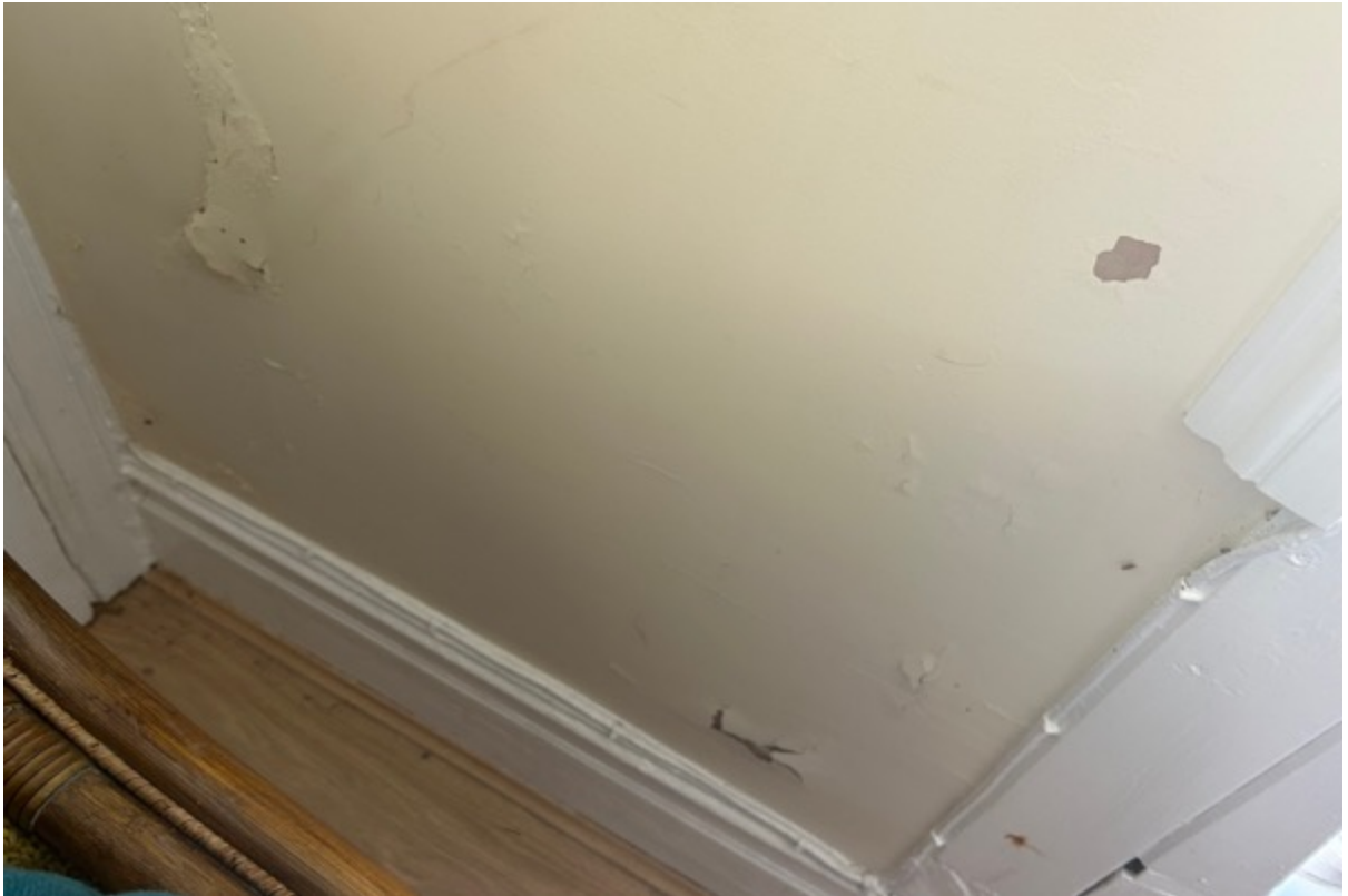
Rising damp to the front wall of the dining area.
