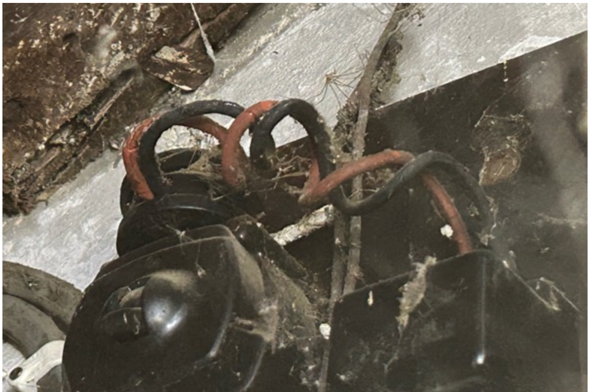
Ancient wiring, with perishing insulation, to the same cupboard.
