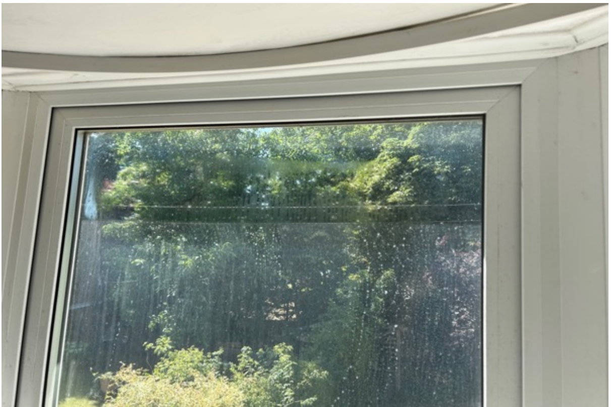
Failed hermetic seal to the front right bedroom window.
