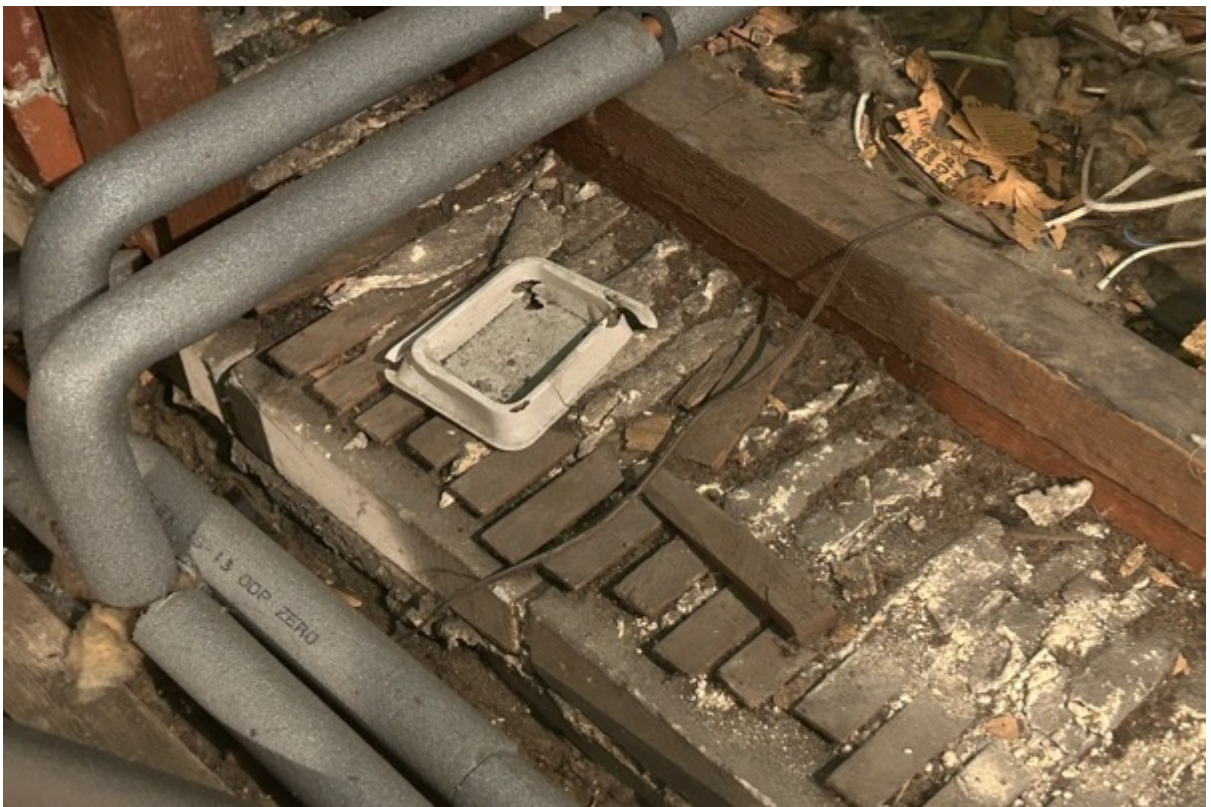
Rodent bait tray within the roof space.
