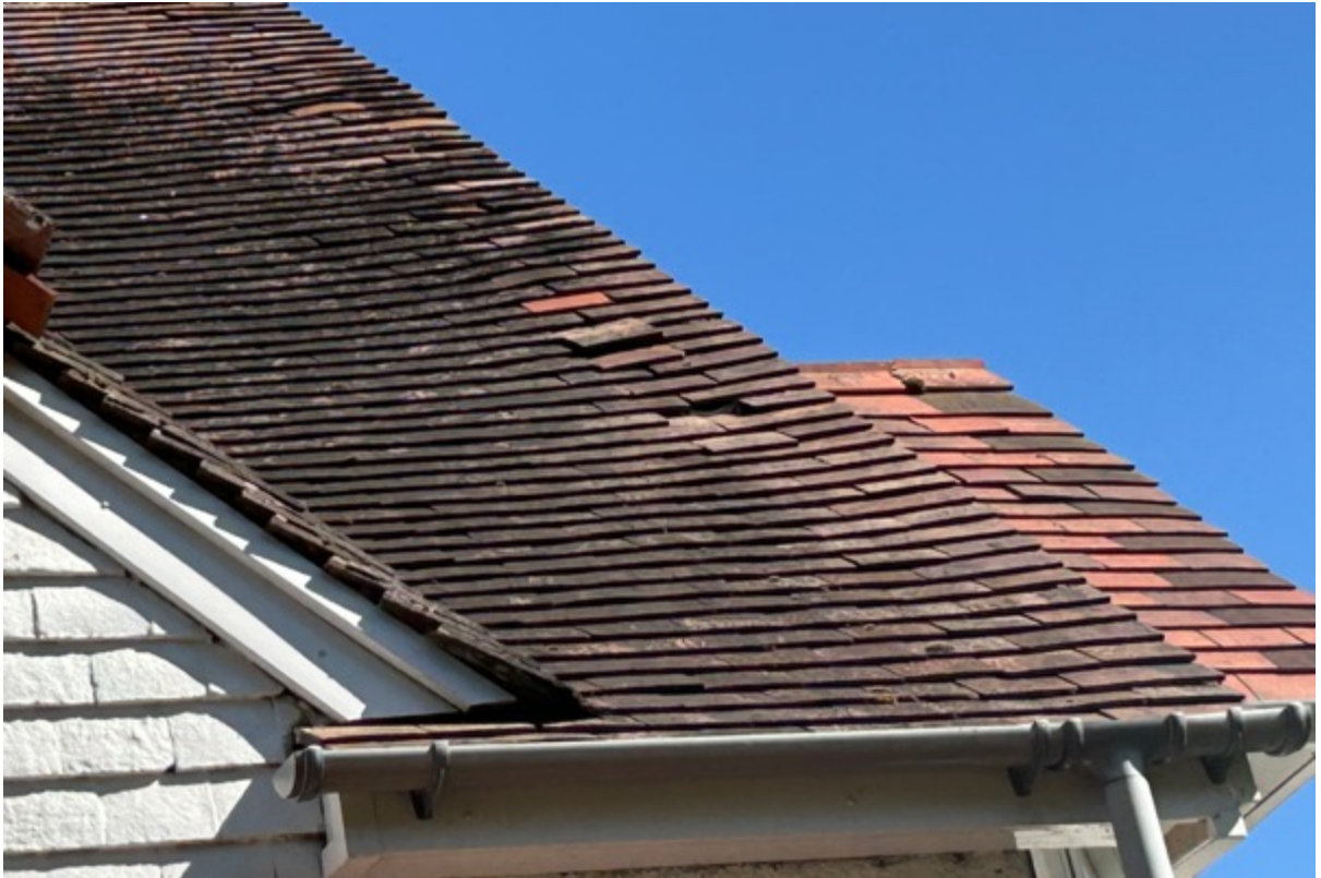
Missing tiling to the right side of the front slope to the main roof.
