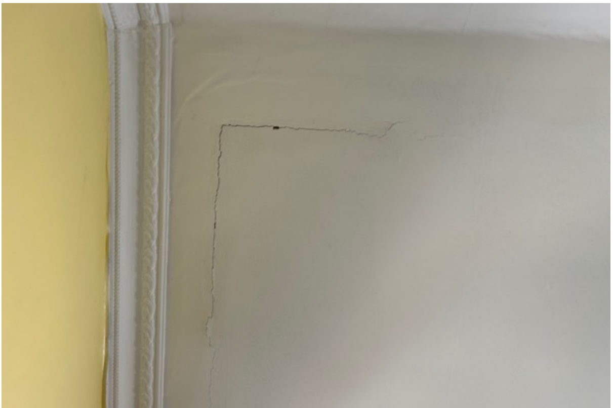
Non-structural cracking to one of the first floor ceilings.
